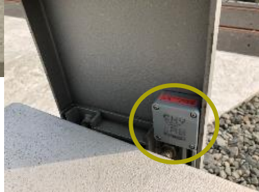
Level crossing sensors
